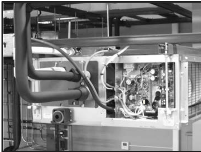
Fan Coil Control PCB
