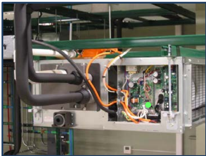
Fan Coil Control PCB
